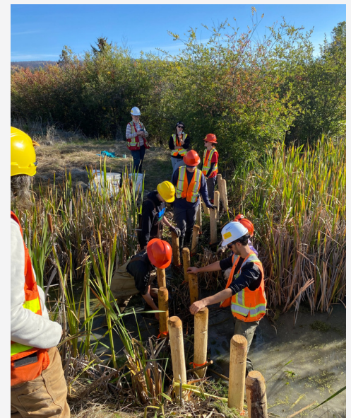
BCIT students constructing a BDA for educational purposes at Logan Lake, B.C.
