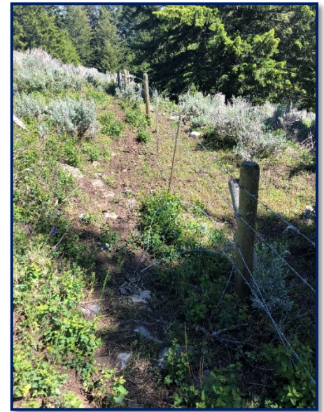
Figure 3. The fencing between the Sawmill Lake and Swartz Creek pastures is not in an effective operating condition. Broken wires allow livestock to freely move between pastures.
